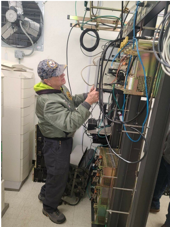
WX2NJ installing the Chatsworth APRS Digipeater
