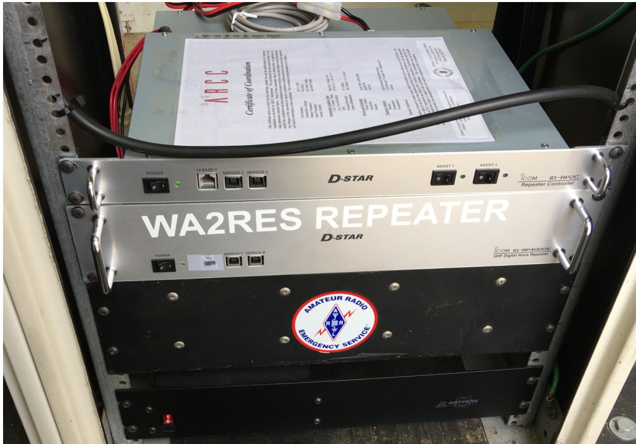
Berkeley D-Star Repeater System
